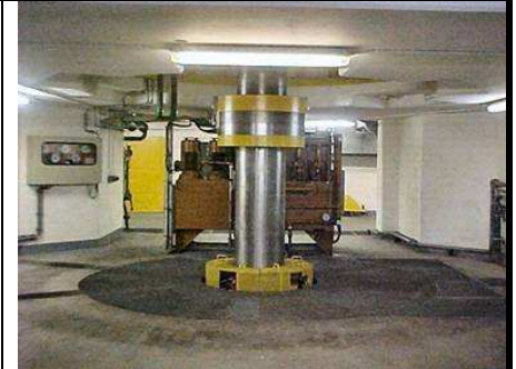
Axel connects Turbine below, to generator above
